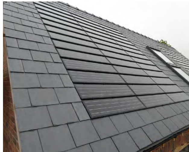
Figure 101: Integrated solar panels on slate roof.
