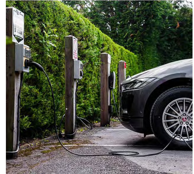
Figure 104: Public electric vehicle charging point.
