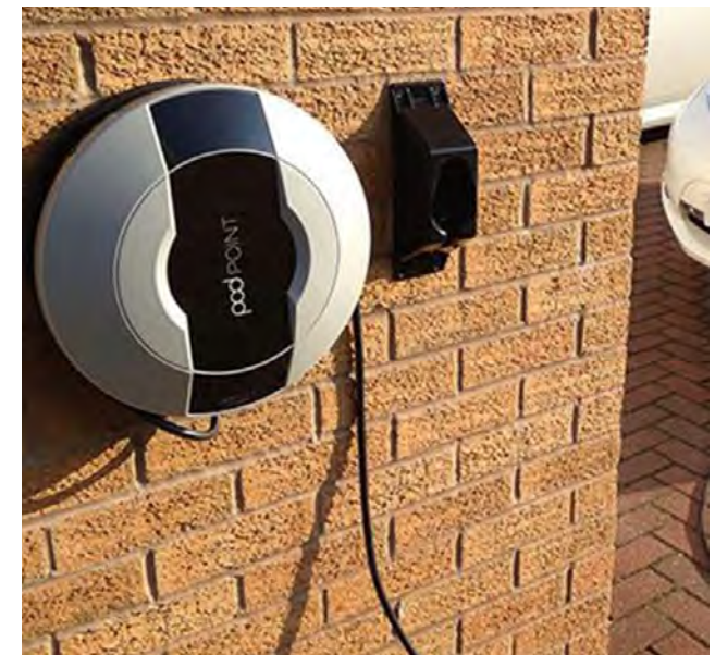
Figure 105: Home electric vehicle charging point.
